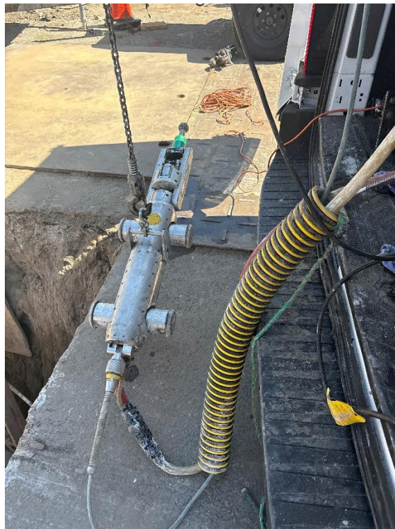
ROBOT FOR PIPE CLEANING
