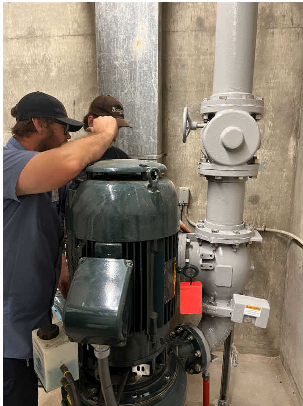
TCWD Operations started Pump No. 1
