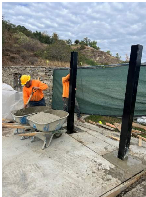
Hemet Fence Company Delivered and Set Posts for Fence Enclosure & Rolling Gate
