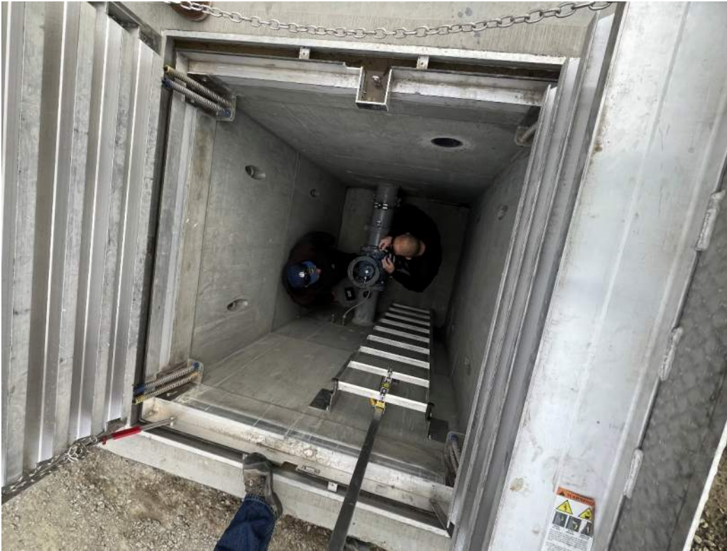
Flow Meter – Testing & Commissioning, by others
