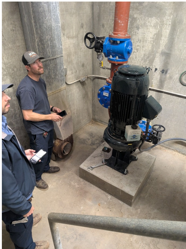
TCWD Operations Performed “Bump Test,” but Circuit Breaker was observed
