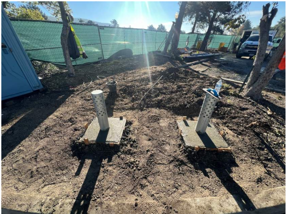
Flow Meter Vault – Complete Vent Piping
