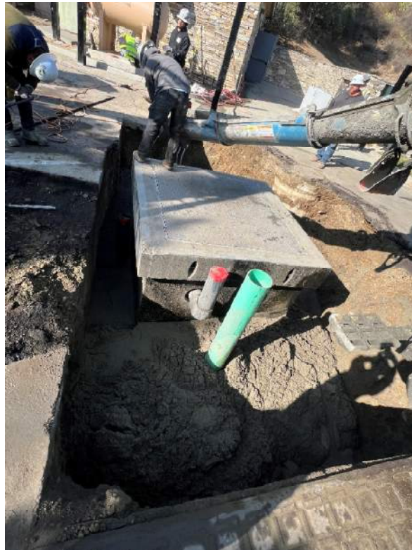
Flow Meter Vault – Slurry Backfill due to Loose Soils; Raise Vent Piping and Valve Can
