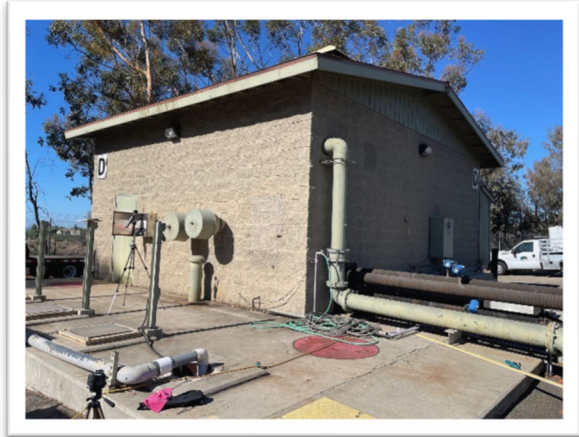
Photograph 1: Existing Blower Building from new pad location. Two existing Hoffman blowers inside structure will be repositioned to new pad.
