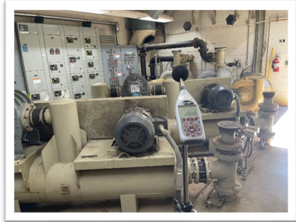
Photograph 2: Existing Hoffman blowers inside Blower Building with Quest/TSI sound level meter.
