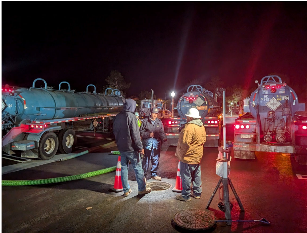
United Pumping Tanker Pumper Trucks In-Place to Collect Sewage Flow During Lift Station Shut Down
