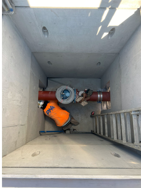
Inside of Flow Meter Vault
