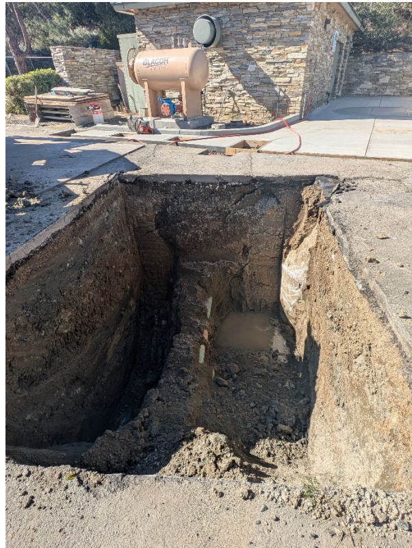
Exposed Epoxy Coated Ductile Iron Pipe of Existing 8-inch Force Main
