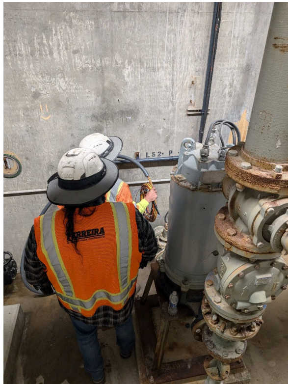
Conduits and Wiring from Upper Level of Dry Pit and Extending into Lower Level of Dry Pit for Pump No. 1
