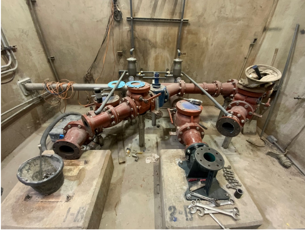
Existing Dry Well – Pump Motors removed and to be replaced; Pedestals to be leveled and improved.
