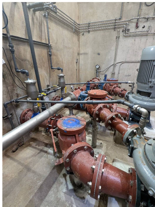
Existing Dry Well – Finished interior of mechanical piping in Dry Well.
