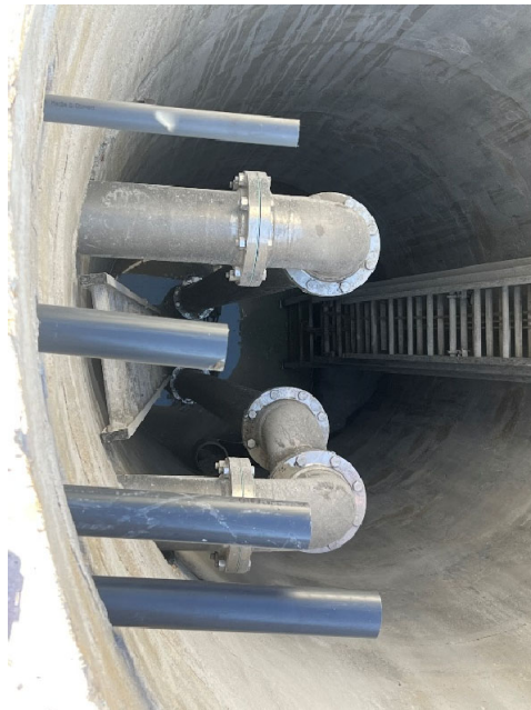
Existing Wet Well – Extension of service conduits inside Wet Well.
