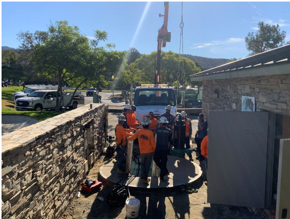
Existing Wet Well – Functional Test while TCWD Operations lifted Submersible Pumps with their equipment.
