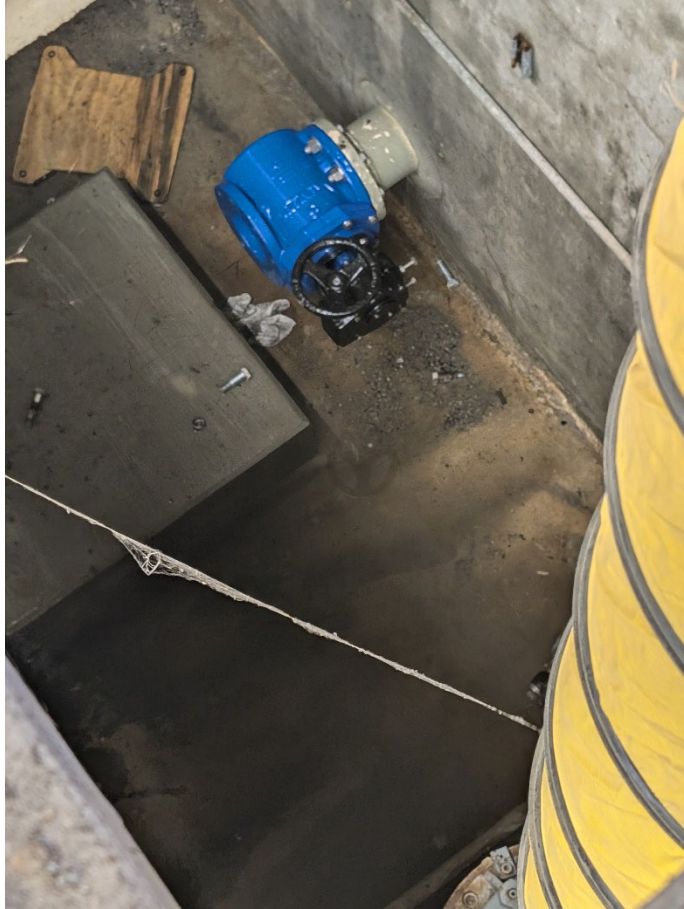
Dry Pit – Installed Suction Plug Valve for Pump No. 1.
