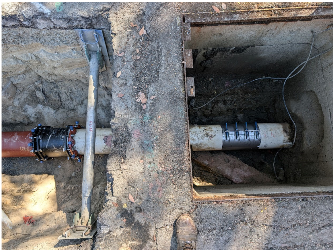
Air Vac Vault – Air Vac Removed, Restraining Band installed; Note: Exposed Electrical Duct Bank.
