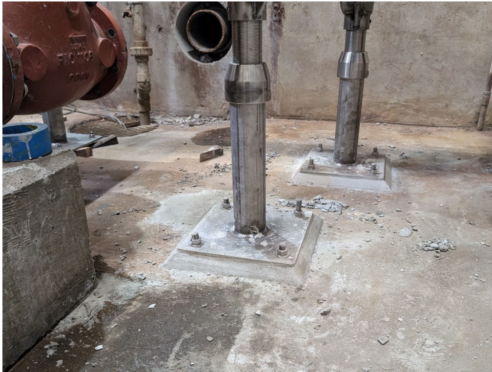
Dry Well – PHC continued with improvements by installing pipe supports and finished with a Rapid Set mortar mix.
