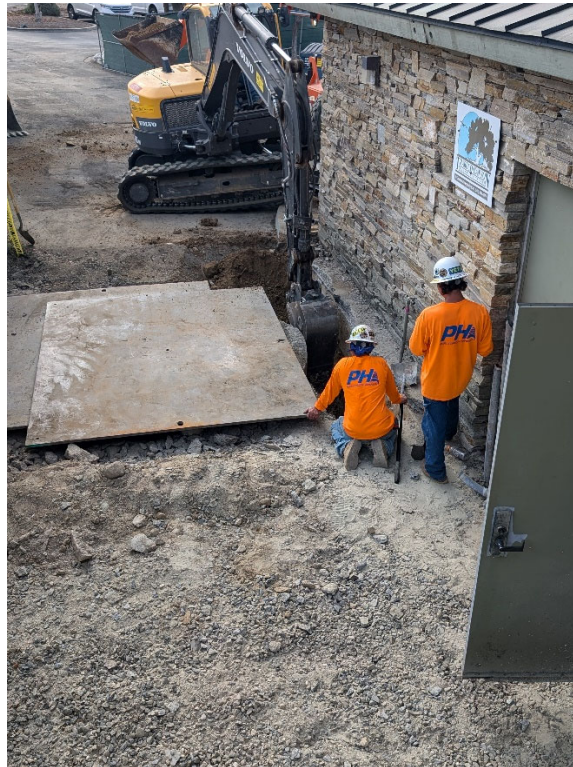
Existing Wet Well – PHC started excavation between Wet Well and Dry Well.
