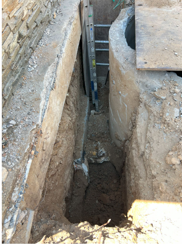
Existing Wet Well – PHC exposed existing pipes between Dry Well and Wet Well and couplings to be demolished and removed.
