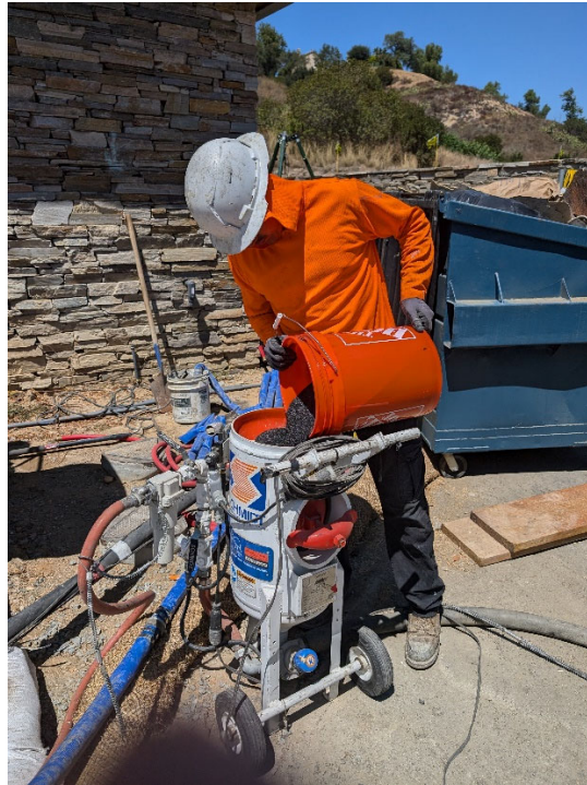
Existing Wet Well – after lining application was removed, TECHNO proceeded to sandblast the interior concrete, wall surfaces.
