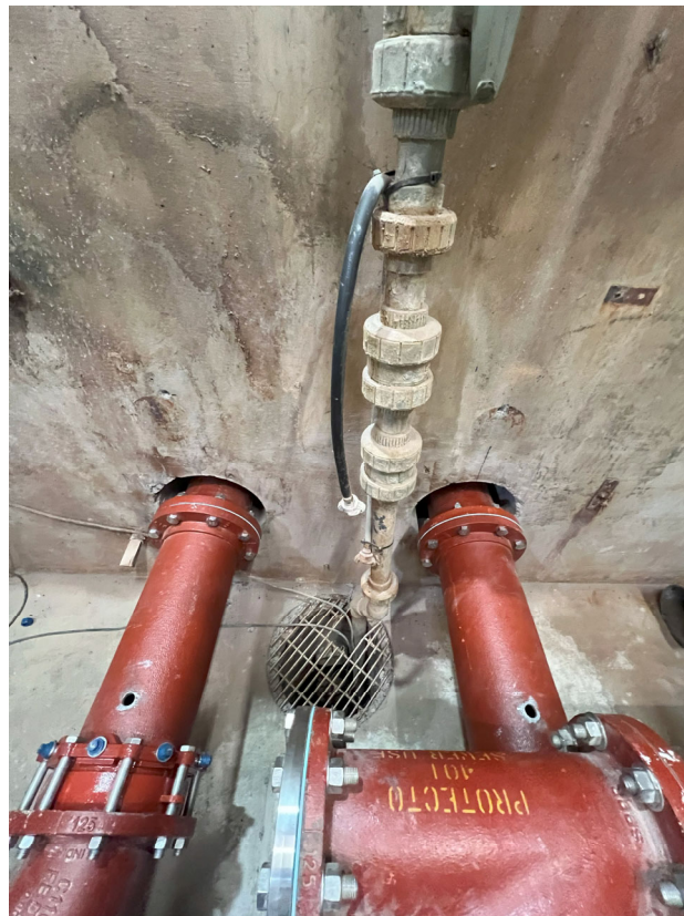
Dry Well – Finished ductile iron pipe spools and connections in Dry Well.
