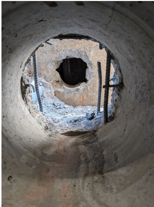
Dry Well – pipe removal, and penetrations from Dry Well looking towards Existing Wet Well.
