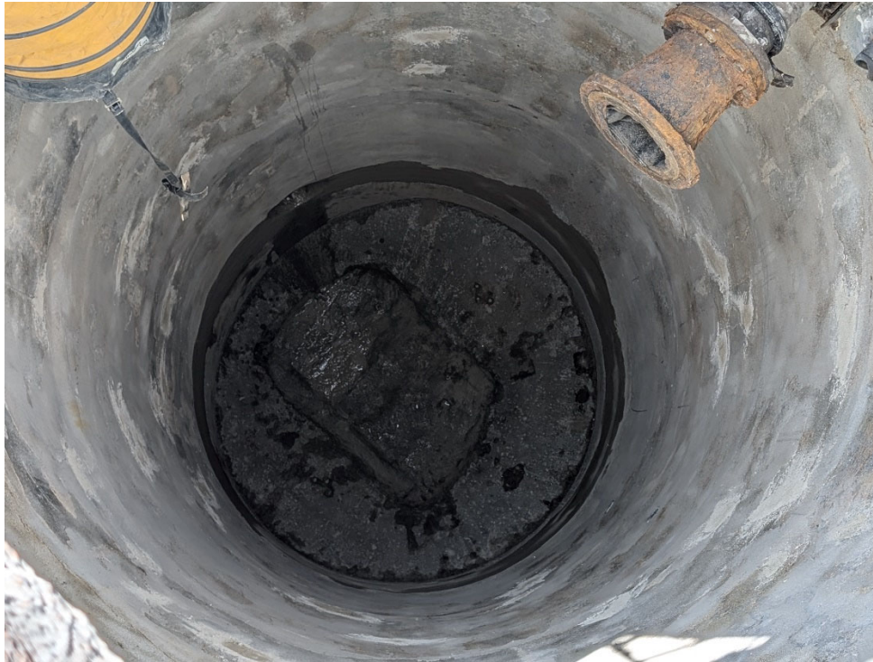
Existing Wet Well – TECHNO demobilized the project site, and cleaned up the bottoms of the Well.
