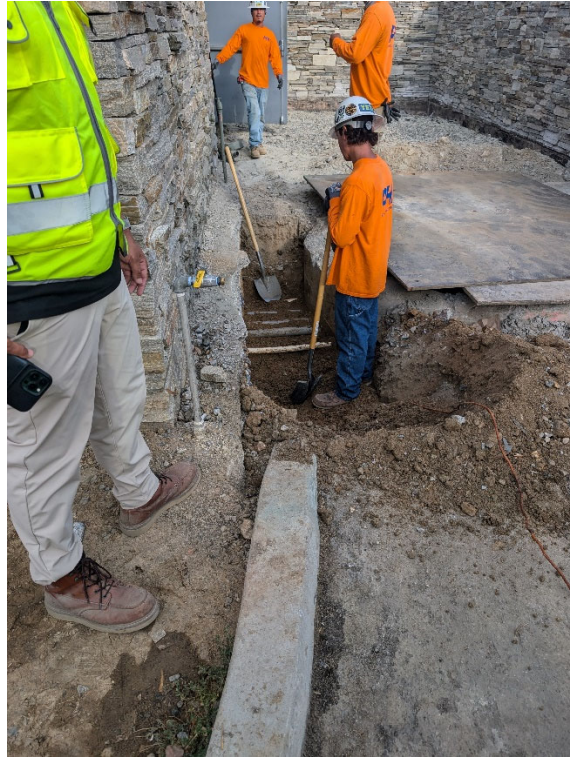
Existing Wet Well – PHC started excavation between Wet Well and Dry Well.
