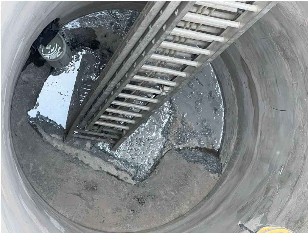
Existing Wet Well – Rapid Set mix to level bottom of Well in preparation for Pump Bases.
