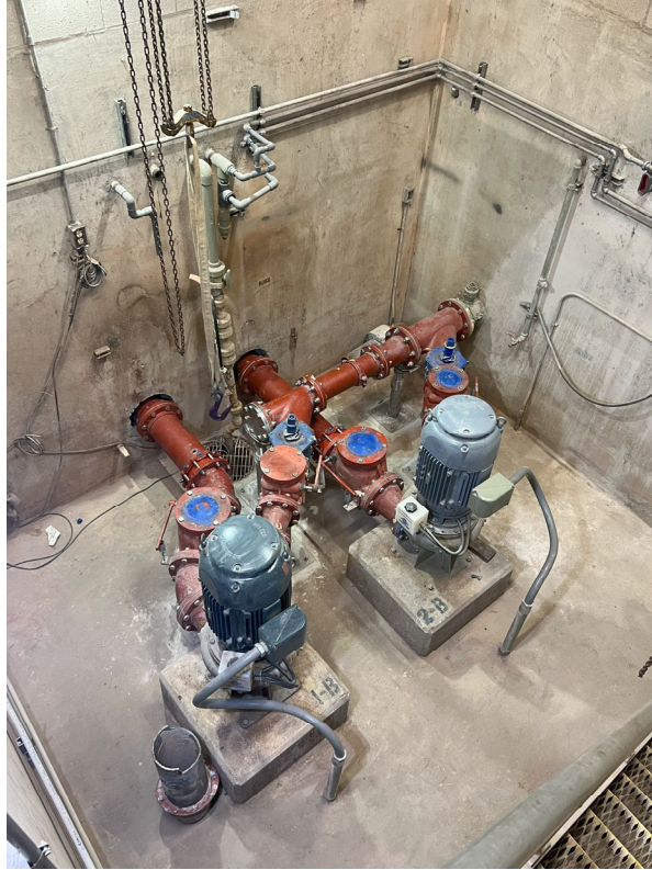
Dry Well – Finished interior of mechanical piping in Dry Well.
