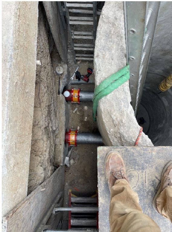
Existing Wet Well & Dry Well – Flex couplings installed and joined dissimilar materials – ductile iron and stainless steel.
