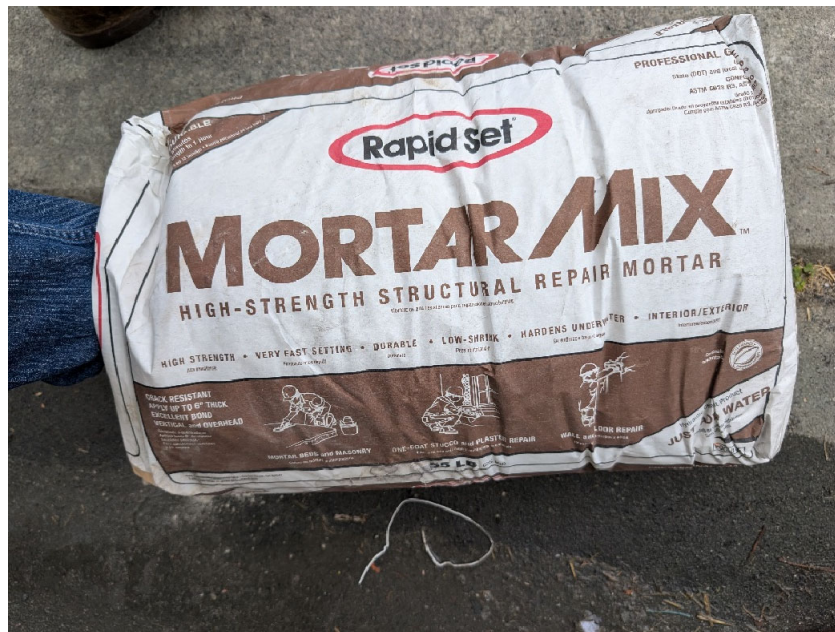
Existing Wet Well – Mortar Mix material used to mix and fill in gaps in the concrete walls.
