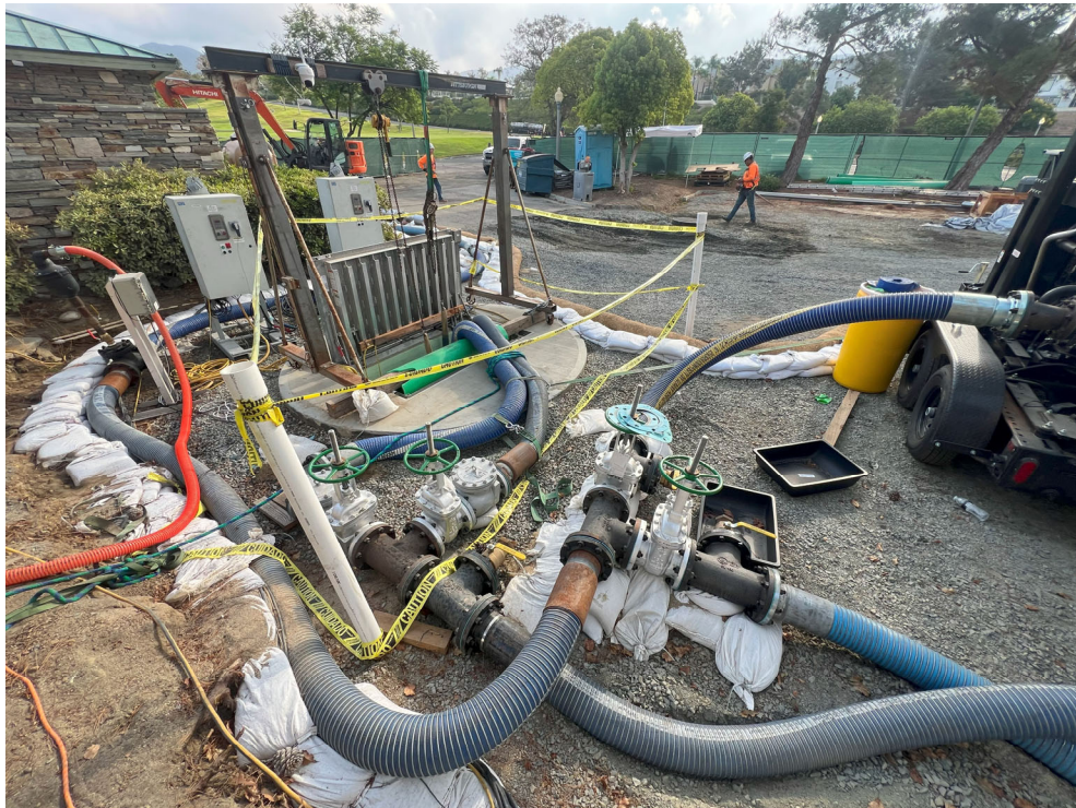
Temporary Bypass System – typical conditions.
