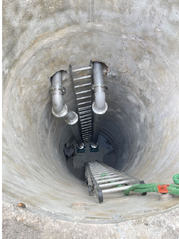
Existing Wet Well – connected and extended stainless steel suction piping.
