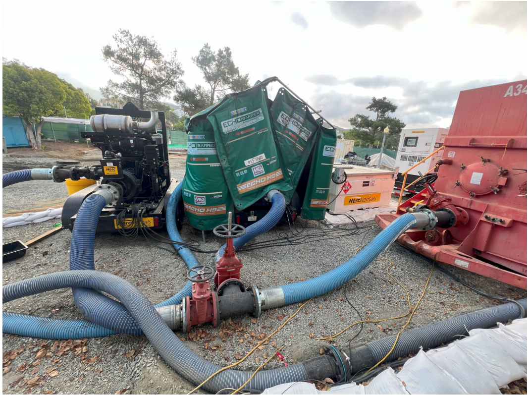
Temporary Bypass System – typical conditions.
