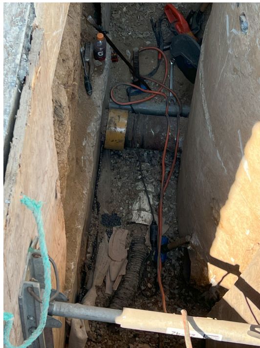
Existing Wet Well – PHC exposed existing pipes between Dry Well and Wet Well to be demolished and removed.
