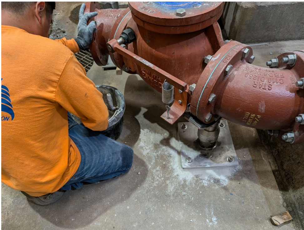
Dry Well – PHC continued with improvements by installing pipe supports and finished with a Rapid Set mortar mix.
