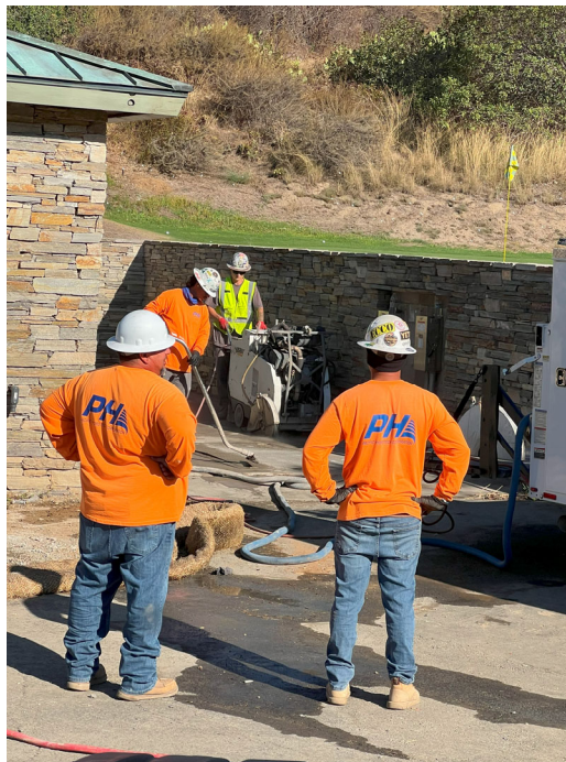
Existing Wet Well – PHC proceeded to sawcut existing finished surfaces at Wet Well to continue with demolition and removals of piping.
