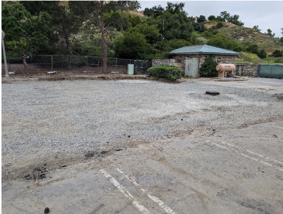
Temporary Demobilization, Project Site – mitigated surface drainage runoff from irrigation into Project Site.
