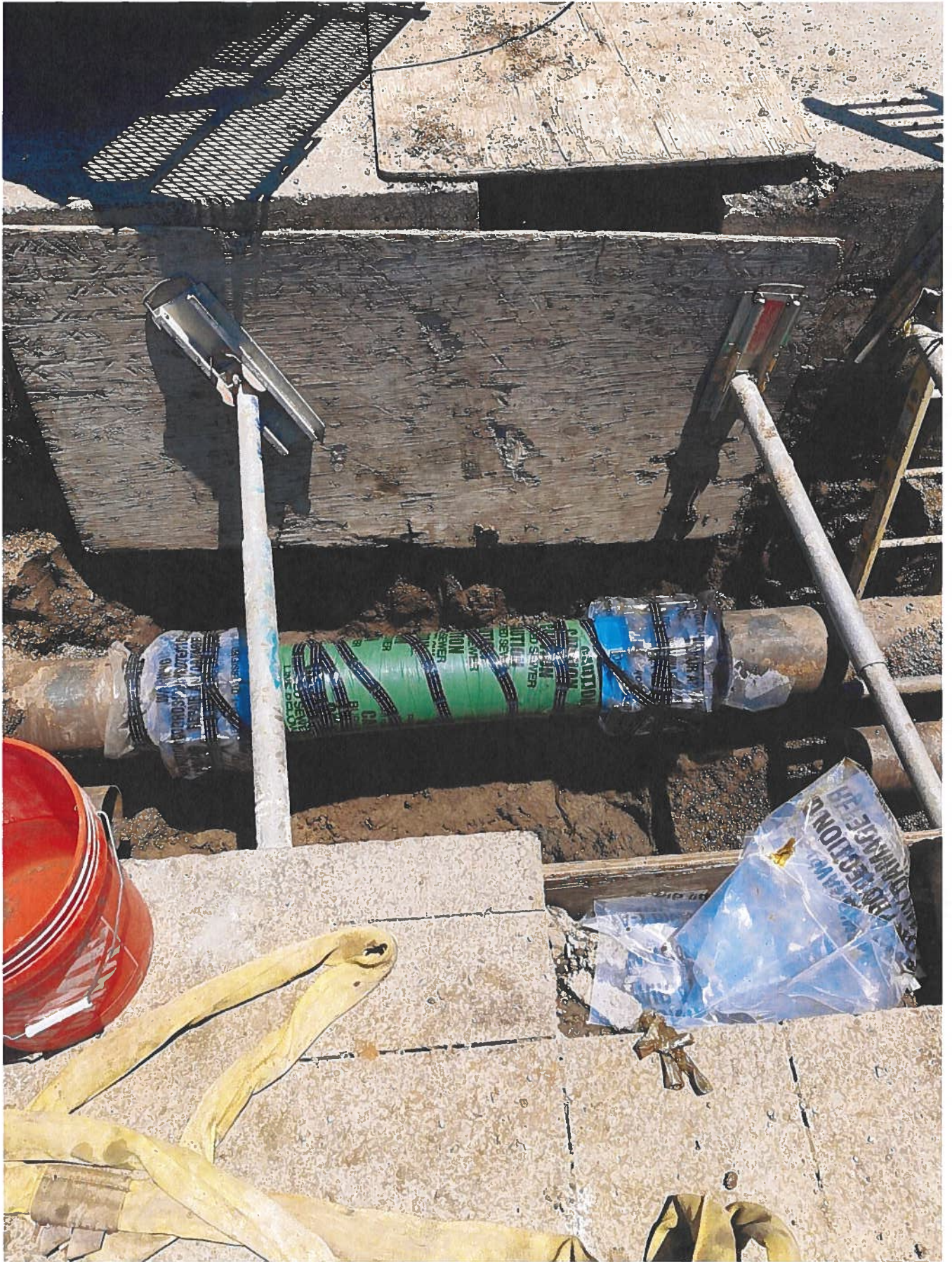
12" Ductile Iron Force Main Pipe Field Repairs Made on June 24, 2024
