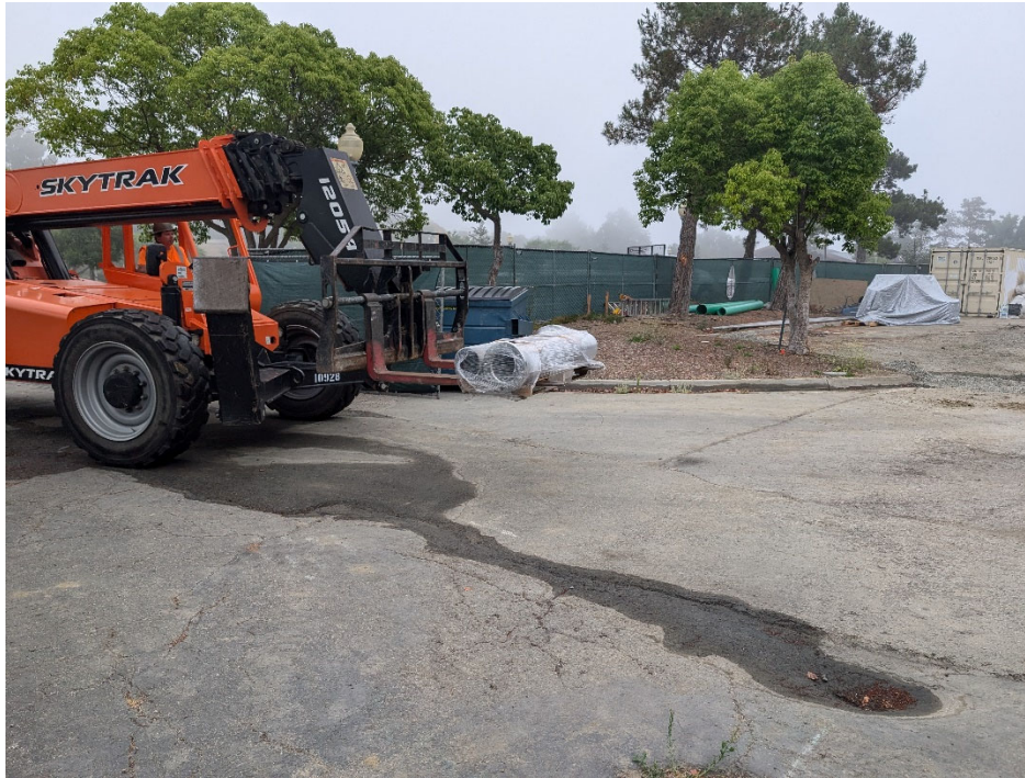
Temporary Demobilization, Project Site – material deliveries. Pumps (covered in tarp) delivered separately by TCWD Operations.
