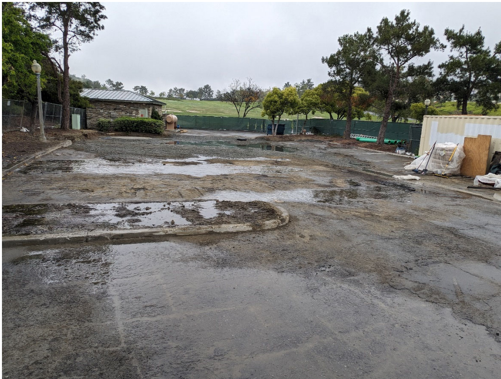
Temporary Demobilization, Project Site – Golf Club surface drainage runoff from irrigation into Project Site.
