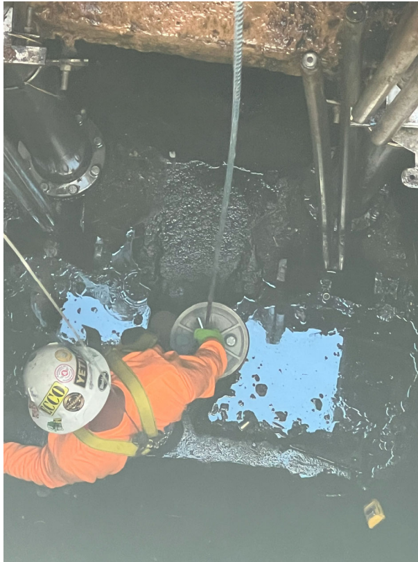
Temporary Bypass System – TCWD Operations given the “Go” to switch over to Temporary Bypass System, and PHC installing mechanical plug for isolation of the Golf Club Lift Station
