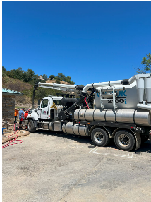
Golf Club Lift Station Demolition – cleanup of Existing Wet Well to start demolition.
