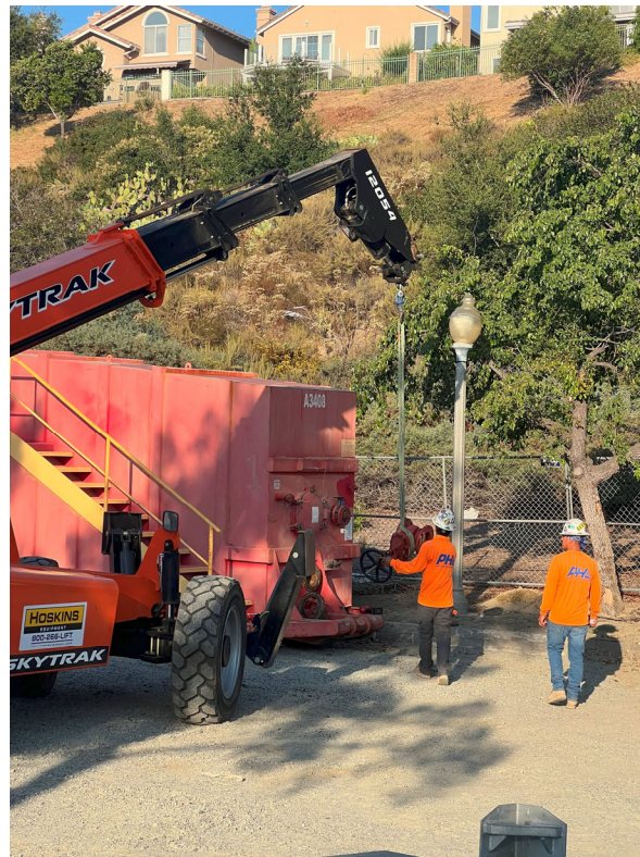
Temporary Bypass System – PHC and HERC Rentals re-mobilized onto the Project Site to start installation of Bypass System.
