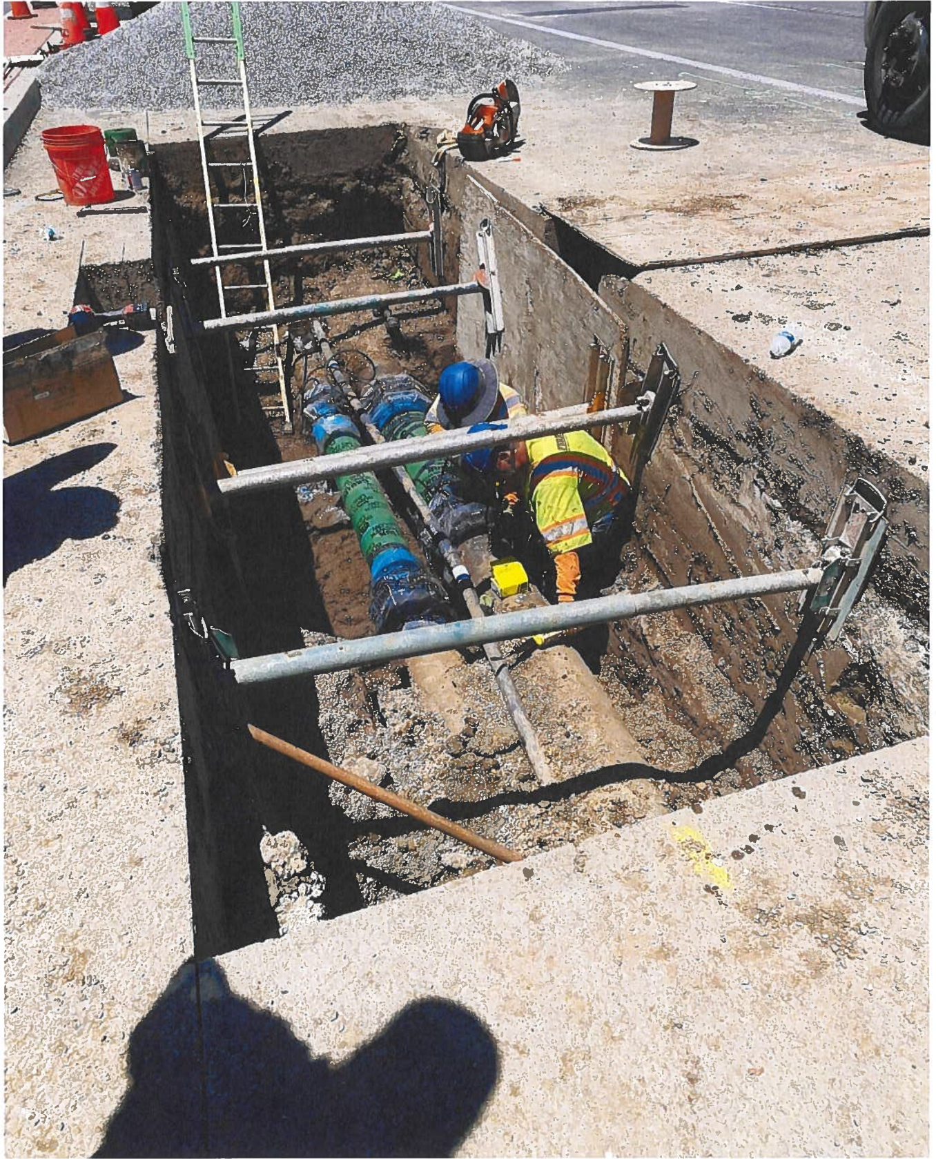
12" Ductile Iron Force Main Pipe Field Repairs Made on June 24, 2024
