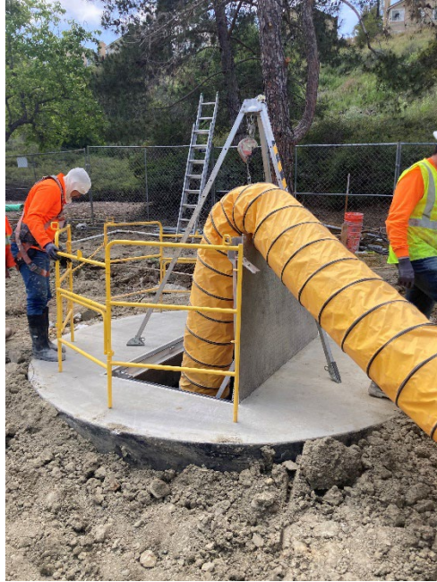
Bypass Wet Well – Techno Coatings continuing to install Raven Epoxy Lining System within the interior of the Wet Well.
