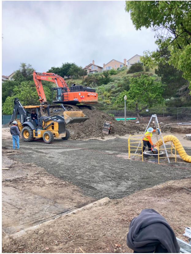
Aggregate Base Material being placed while Techno Coatings is lining the Diversion Manhole.
