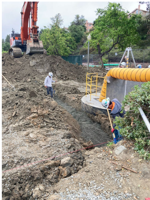
Unmarked Domestic Water Line – placement of bedding material and identification tape prior to Aggregate Base Material placement.
