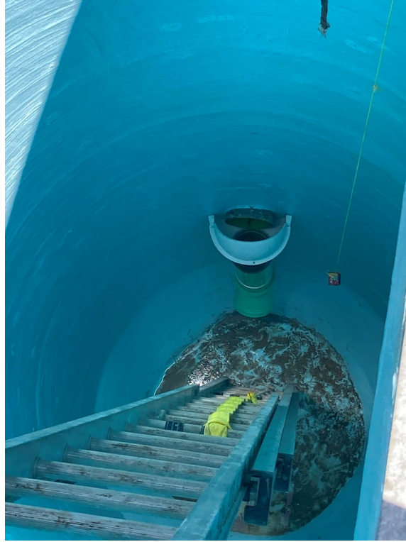
Bypass Wet Well – PHC installed Overflow Pipe.
