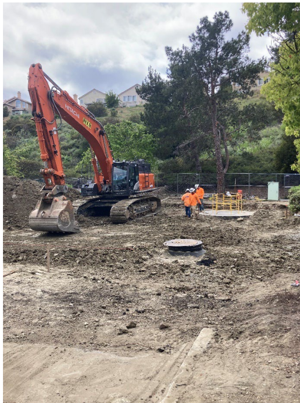
PHC continuing to place and compact subgrade materials around the Bypass Wet Well and Diversion Manhole.
