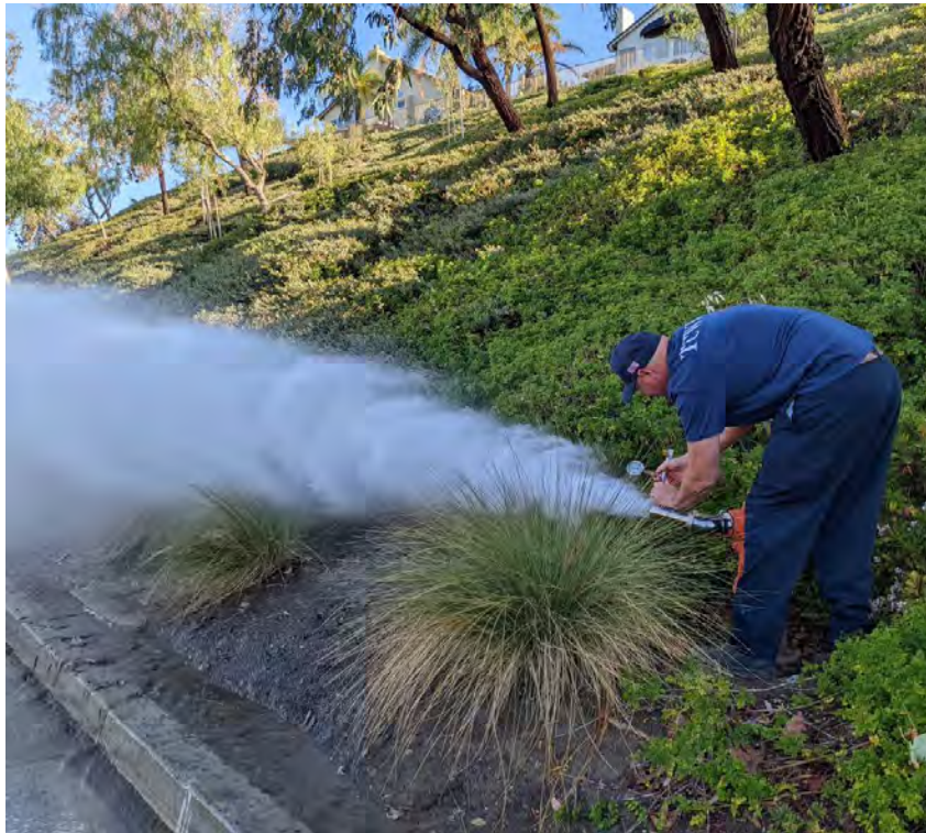
Figure 5-1: Fire Flow Test – Flow Hydrant
