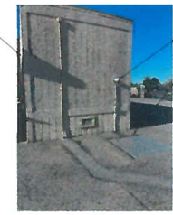
FLOW METER TRANSMITTER PHOTO 3 NTS
