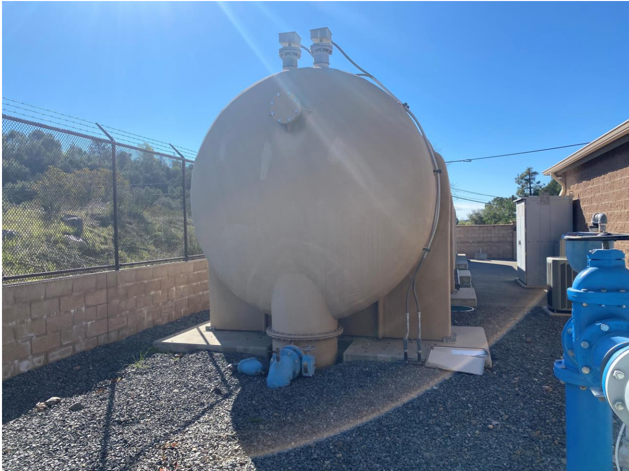
Figure 2-3: Chlorine Contact Tank
