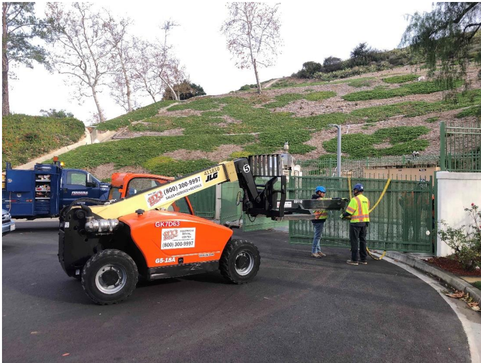
FERREIRA Removing Existing Swing Gate to Replace Perforated Metal Screen and Powder Coat
