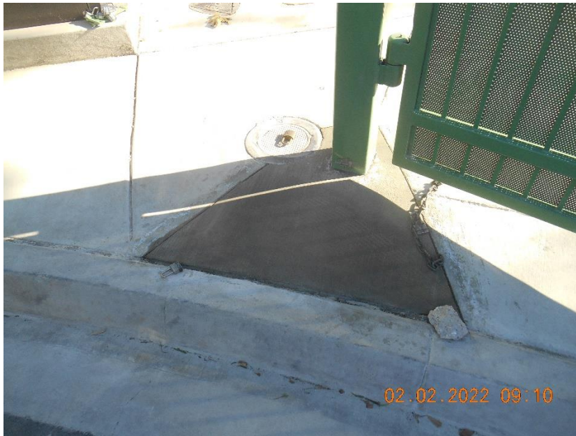
Concrete Apron Remediation Complete Around New Post – Broom Finished to Match Existing
