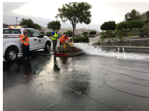
Moulton Niguel Water District staff conducting hydrant test with Hazen team member
