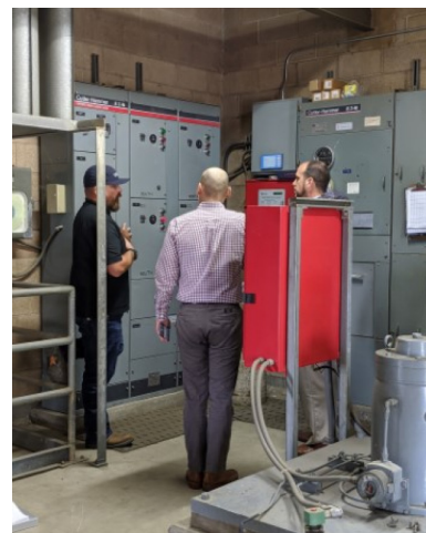
Hazen electrical engineers discussing El Toro Lift Station with Jason Stroud.
