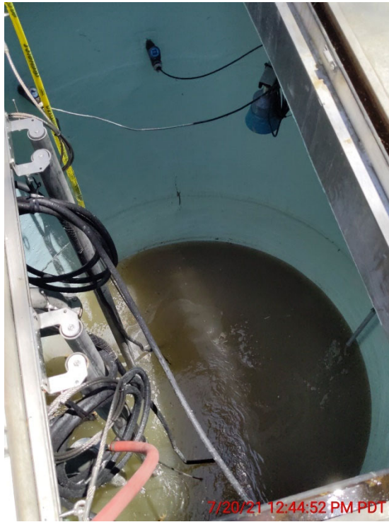
Status of 48-Hour Functional Testing up to (7) Day Acceptance Testing
