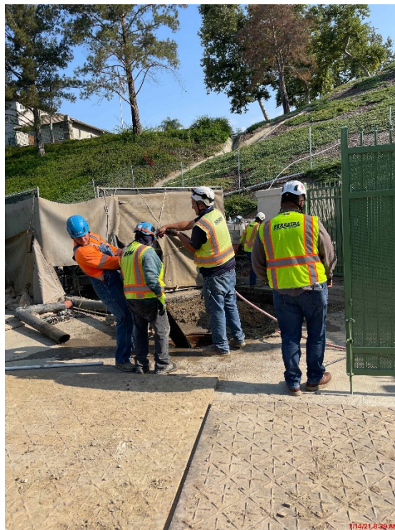
Start-Up of 48-Hour Functional Test of Lift Station
