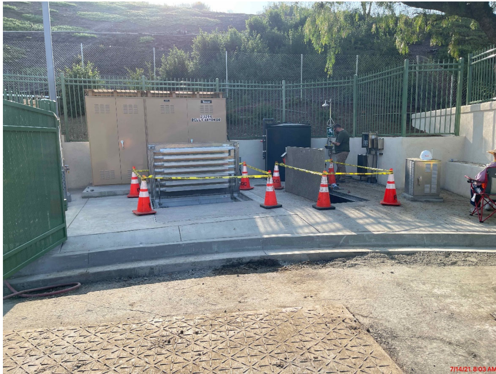
Start-Up of 48-Hour Functional Test of Lift Station
