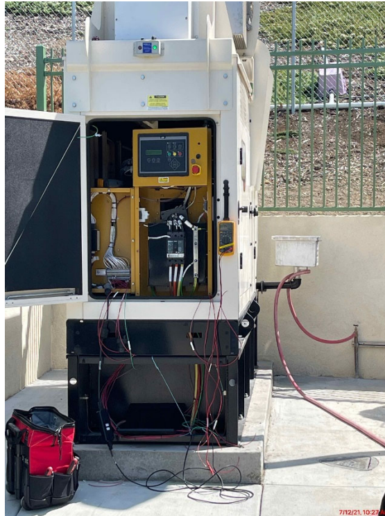
QUINN-Caterpillar Generator Field Testing
