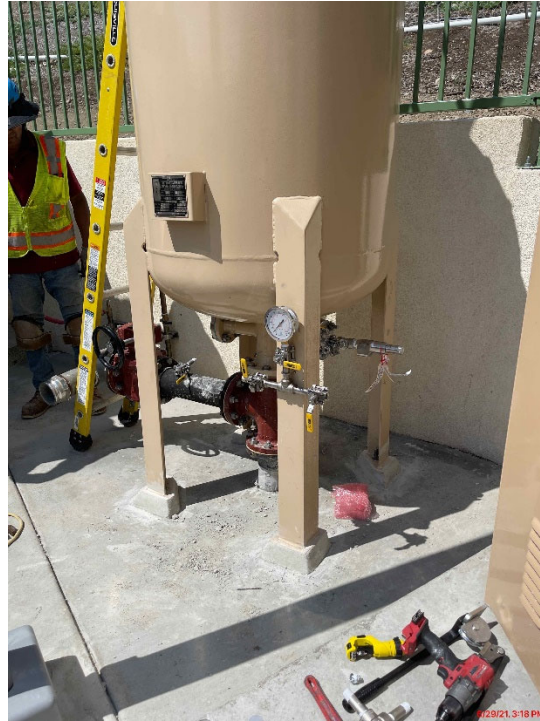
Surge Tank Being Tested
