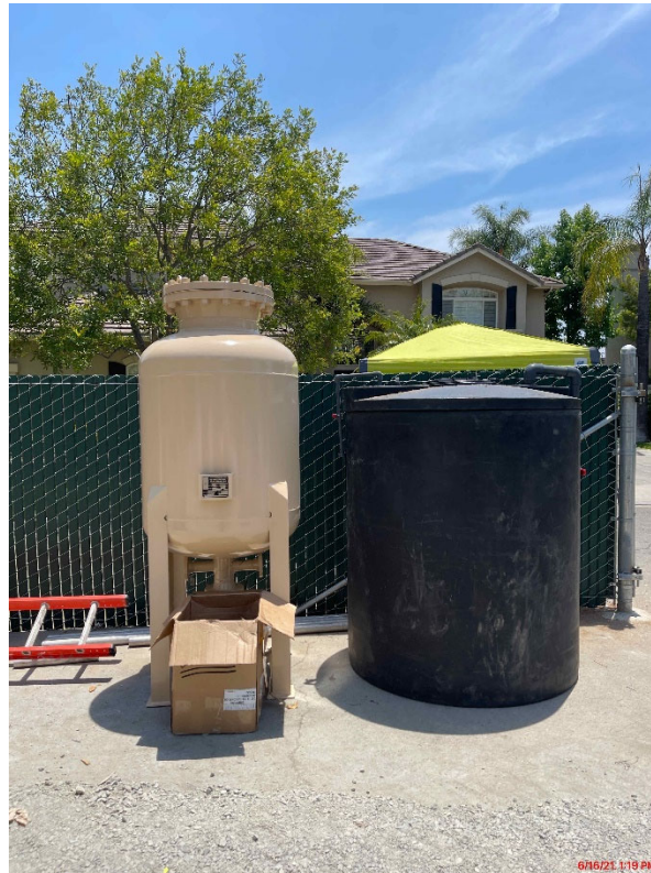
Surge Tank & Chemical Feed Tank Delivered to Lift Station
