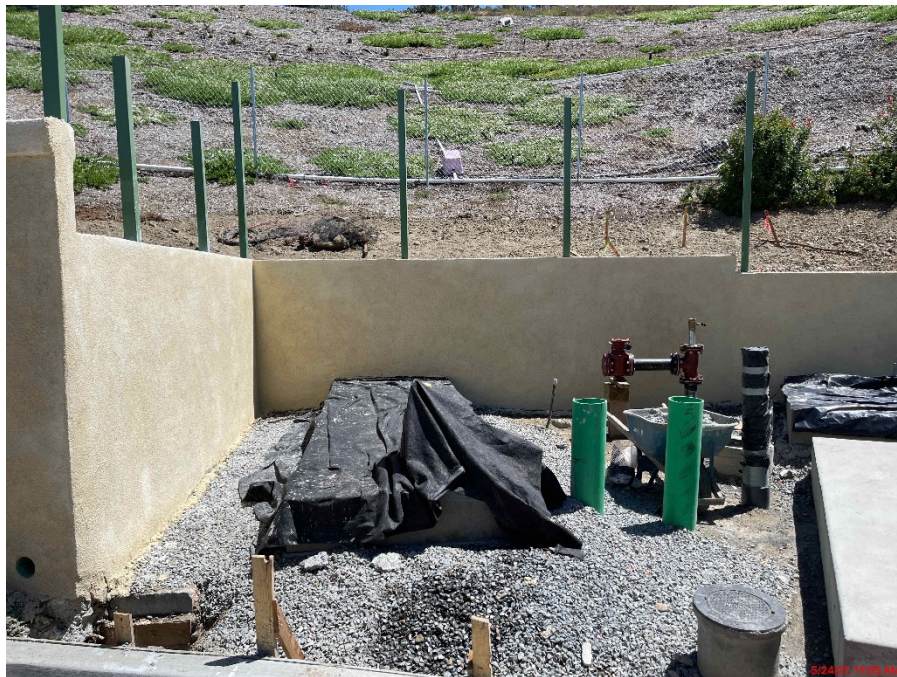
Stucco color and finish of new and existing Walls; and Wrought Iron fence post installation
