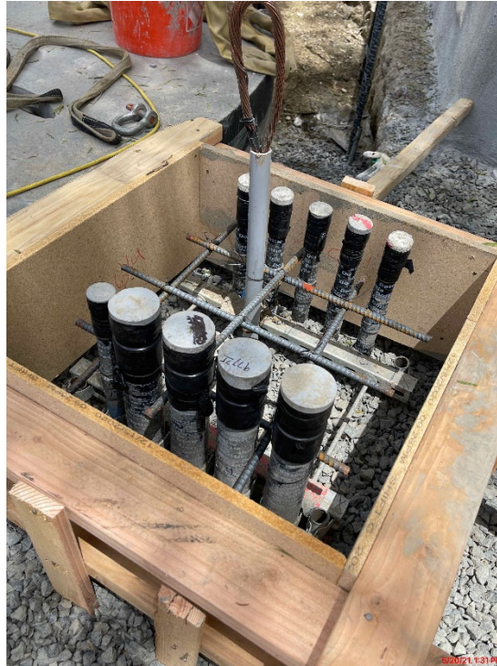
Form Sump Termination Pad
