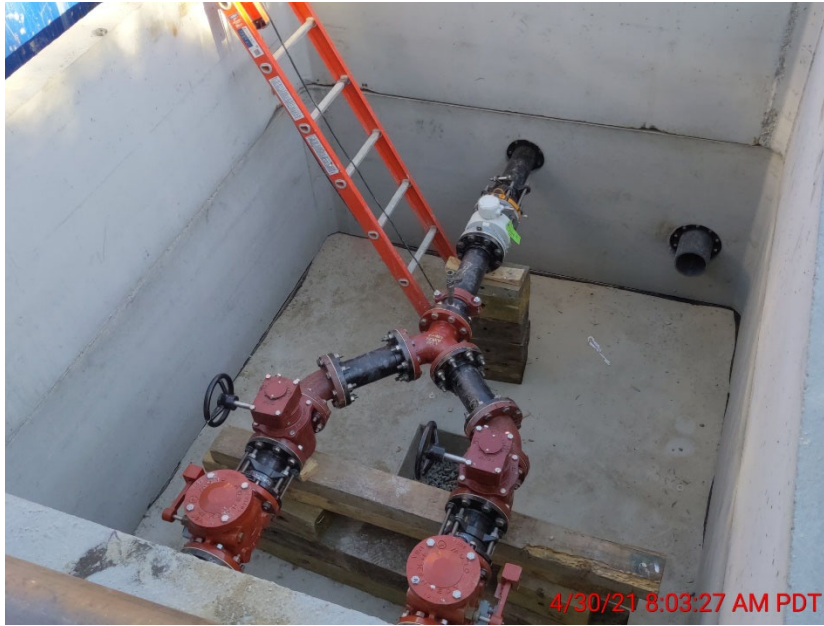
Mechanical Piping in Dry Well Vault
