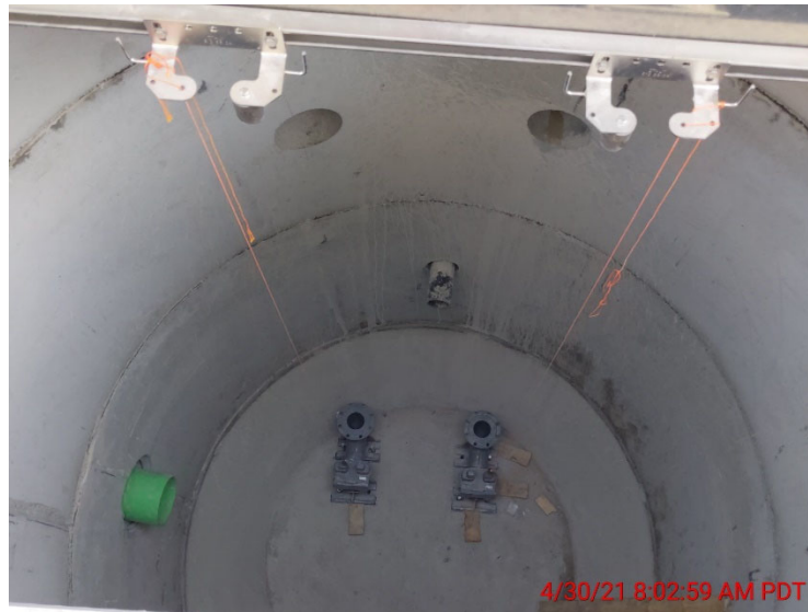
Submersible Pump joints at bottom of Wet Well
