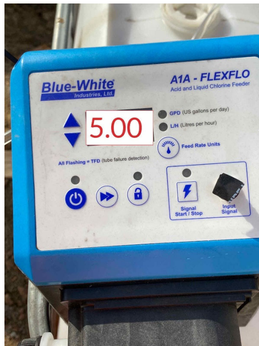
Dosing Meter for Odor Control
