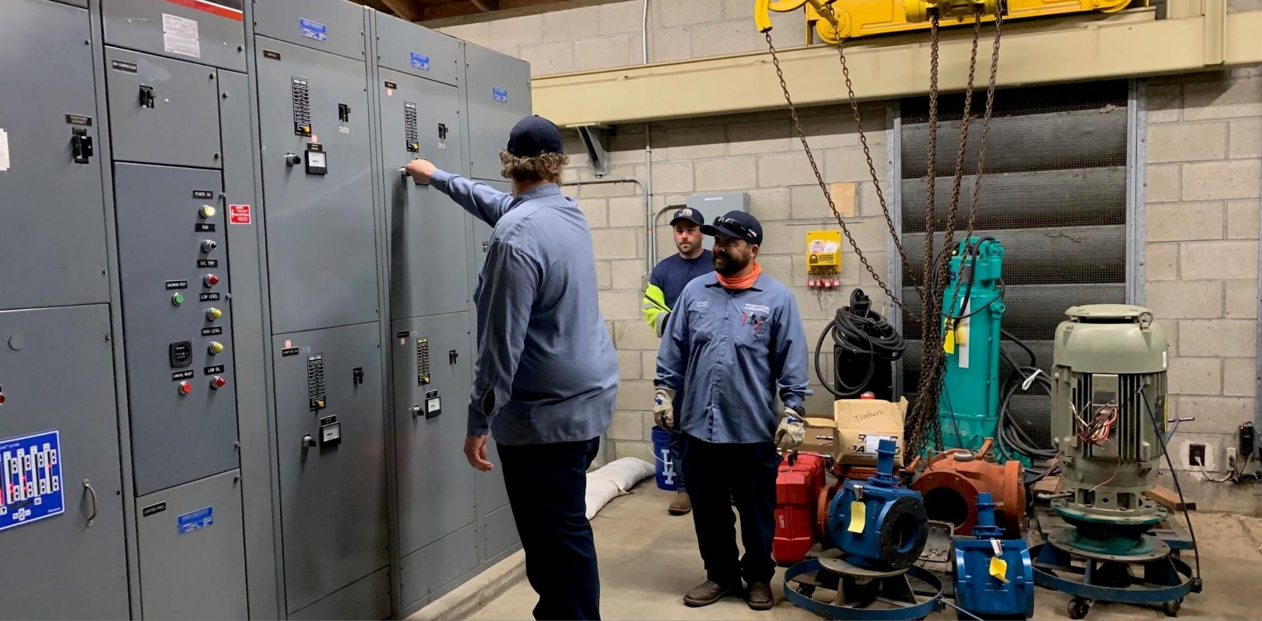
O/M Staff performing Lock Out/Tag Out on station pumps
