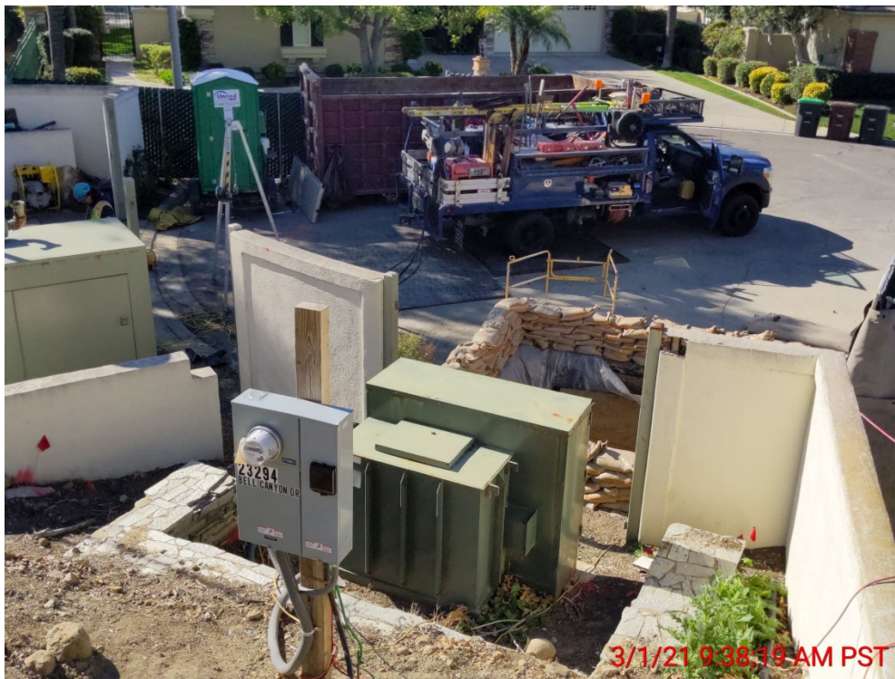
Temporary Panel (foreground) to support Switch Over
