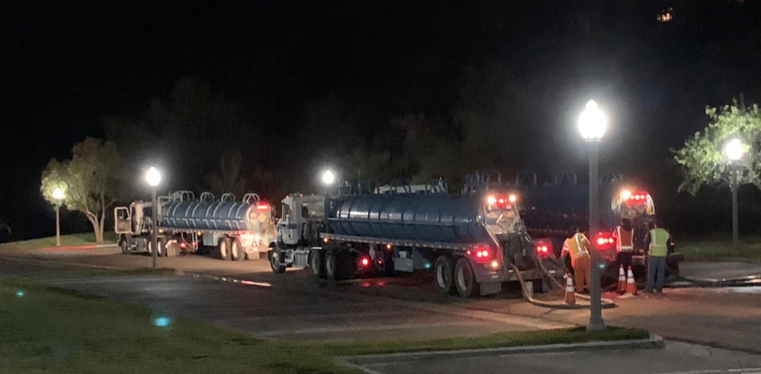
Three pumper trucks collect wastewater flow upstream from the station.
