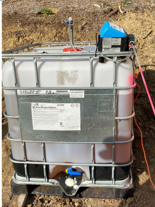
Nitrate Dosing Tote for Odor Control
