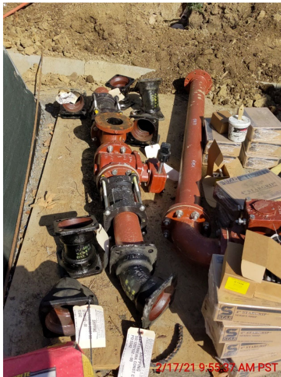
“Cut-In Valve” system
