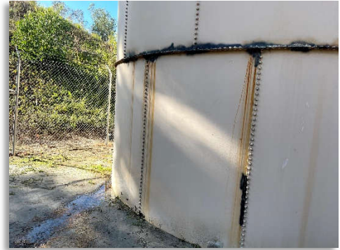
Photo 2 – Corroded Shell of Southerly Backwash Settling Tank
